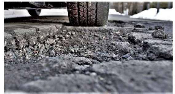
Excessive shock loading from potholes / curb impact
